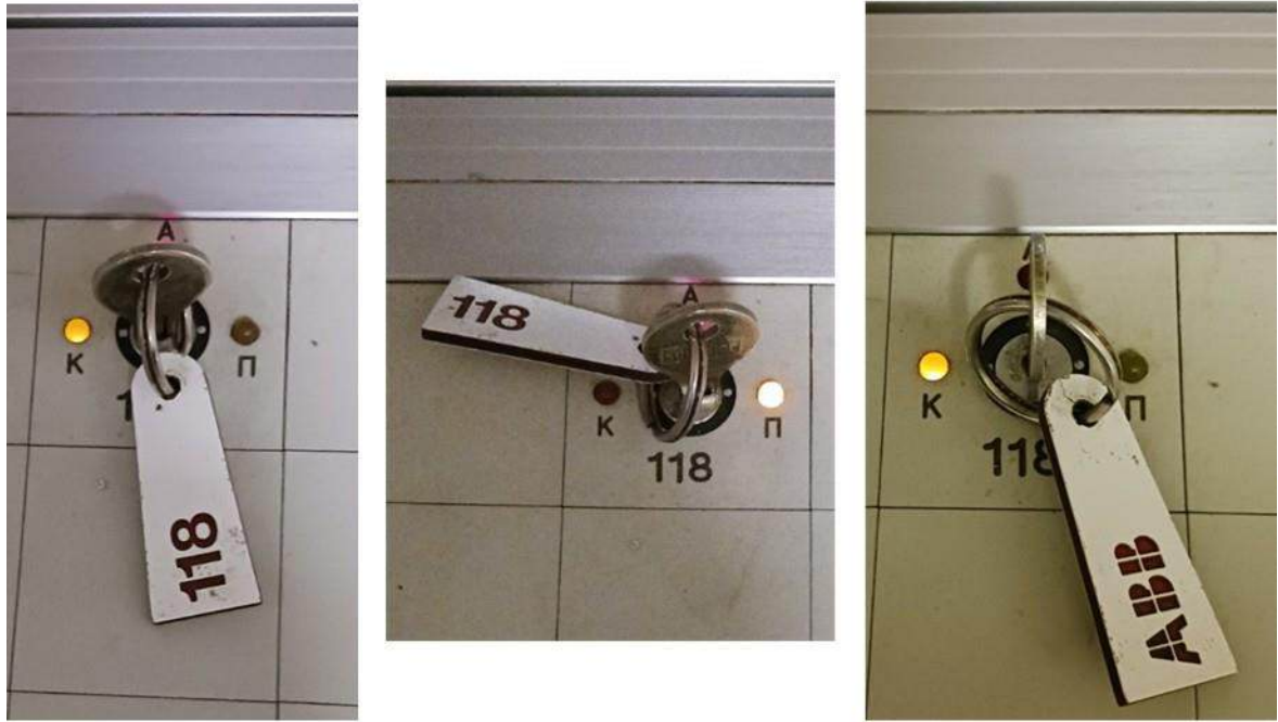
Figure 46. Detail of the three-position key for handling switches 118 on the Larissa Control Panel.
